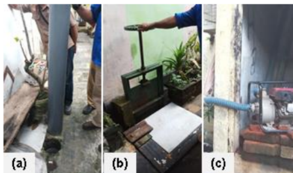
Figure 3. The existing flood resilience system consists of water level indicators at subsurface sewer (a), sluice gates for controlling water level (b), and pumping stations to raise water to the nearest receiving water body (c)
