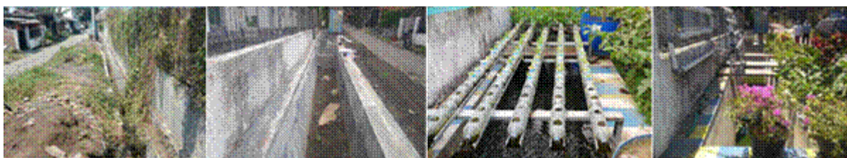
Figure 2. Transformation of the study site, starting before the drainage channel improvement project, the construction phase, modification of the channel for fish and vegetable cultivation.
