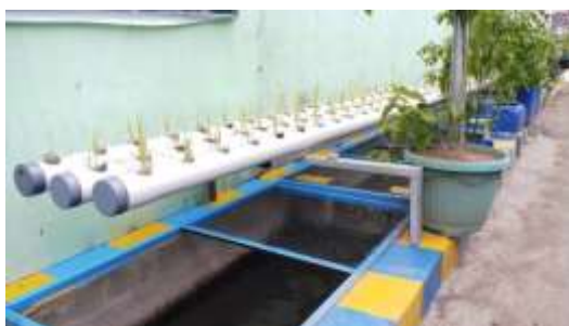
Photo 2. Retrofitting the drainage channel for fish cultivation, and water reuse for vegetable cultivation
